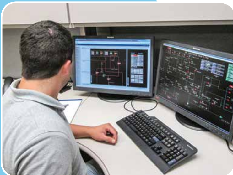
Human-machine interface and distribution automation EMS screens aid with routine operations. Photo courtesy of SEL
