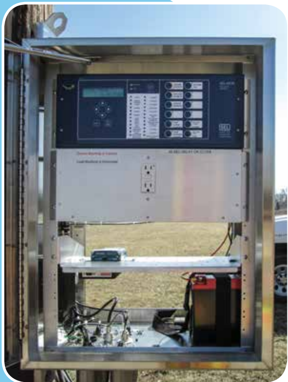
System components include advanced recloser control, satellite-synchronized clock, and wireless 3G cellular modems. Photo courtesy of SEL
