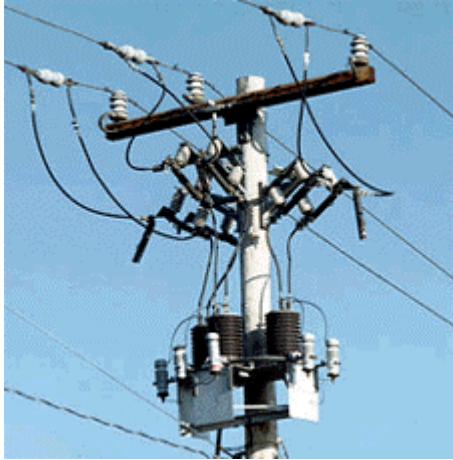
A transformer on a utility pole
