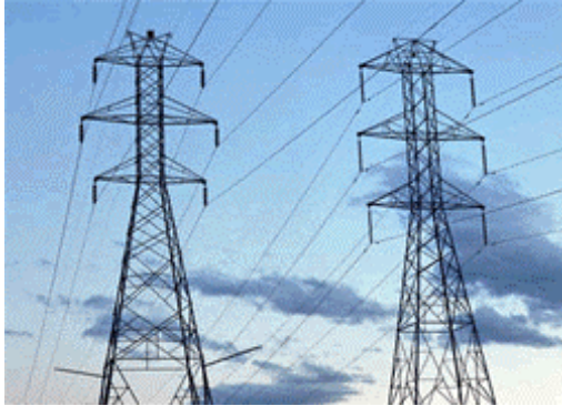
Power transmission lines
